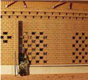
Masonry detailing - 'missing block'
